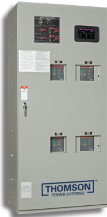
800A TS870 Bypass, 4 breaker configuration
